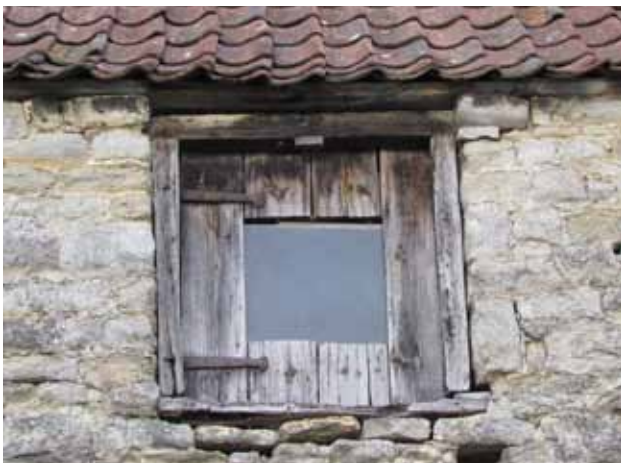
Window in a building at Kelston Mills Rory Walsh © RGS-IBG Discovering Britain
